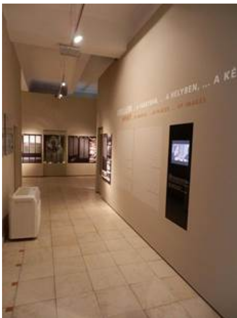
4.27. picture: An air conditioning device in an awkward position in a narrow museum corridor. (Photo: Tamás Vásárhelyi)
