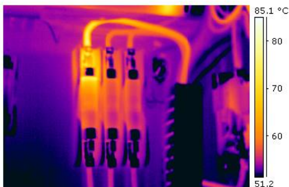
Figure 1.11: Thermogram of an industrial electrical fuse block with a fault (bright yellow area) http://en.wikipedia.org/wiki/File:Electrical_fault.jpg
