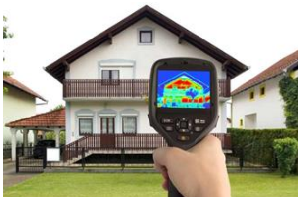
Figure 1.12: Thermography – or infrared scanning – in use to detect thermal defects and air leakage in building envelopes. http://energy.gov/energysaver/articles/thermographic-inspections
